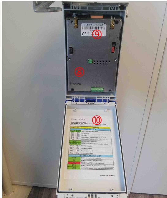
Figure 6 : LoRa IoT Station casing - internal view
