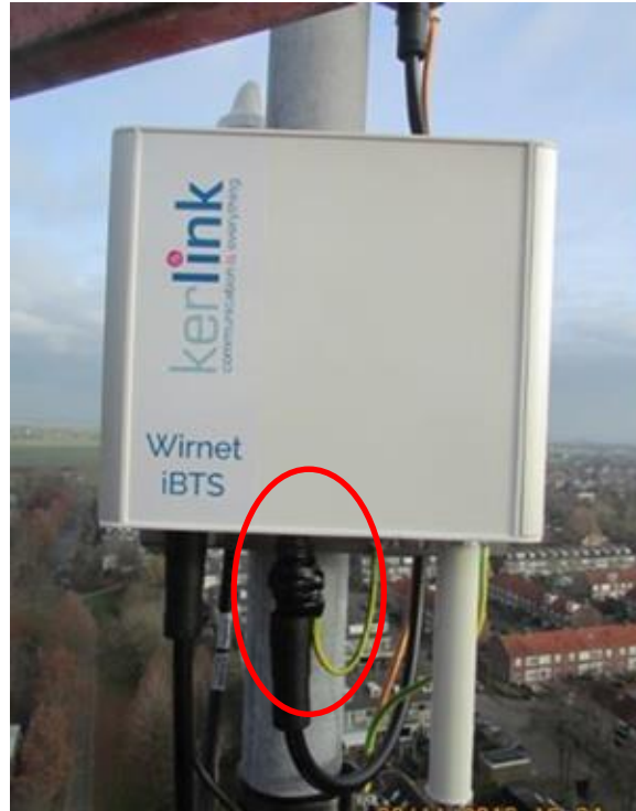
Figure 50 : Example of insulating tape protection on Wirnet iBTS gateway RF port with coaxial lightning protection
