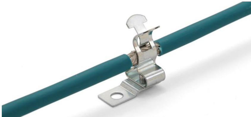
Figure 65 : Earthing of the Ethernet cable
