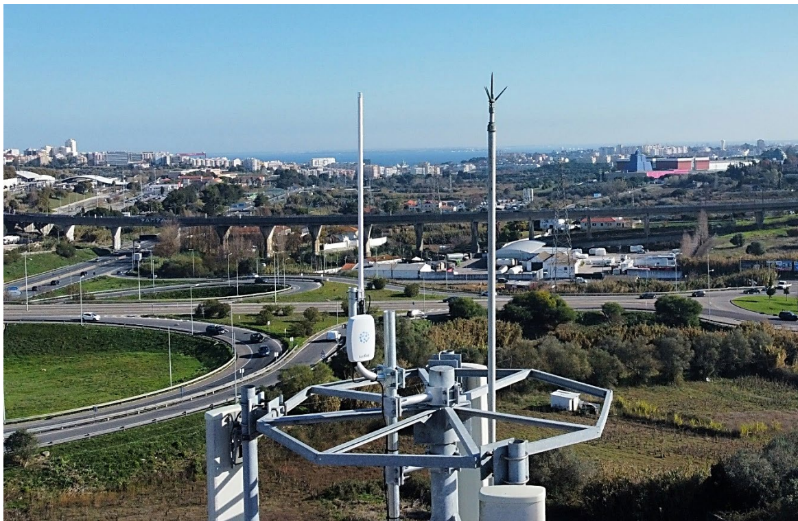
Figure 15 : Installation on top of a tower, with lightning rod - @Lorin, 2021
