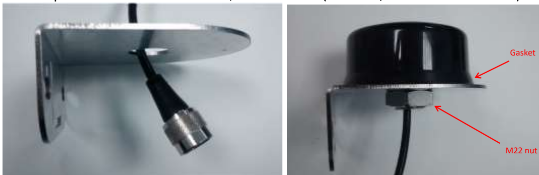
Figure 24 : N connector introduced in the hole of the dome antenna bracket / Figure 25 : Antenna installed on the dome antenna bracket
